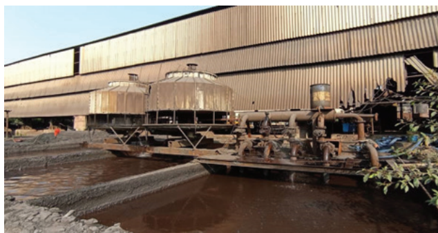
Water pumping system in SRRM
