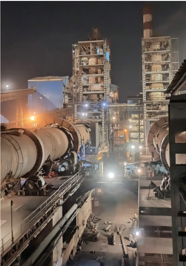
View of DRI plant
