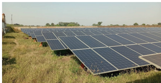
Ground-mounted solar PV system already installed at one SRRM unit
